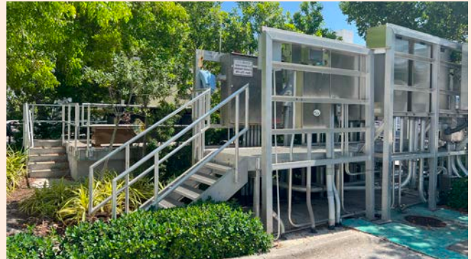
Elevated stormwater pump station and electrical panels. Source: Miami Beach
