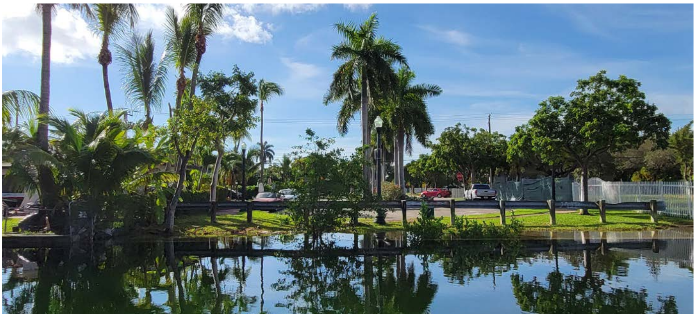
King tide floodwaters overtopping canal seawall in Miami Beach. Source: Miami Beach
