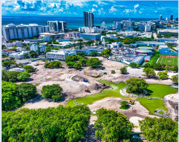
Aerial photo showing the construction of Bayshore Park and retention lake Source: Miami Beach
