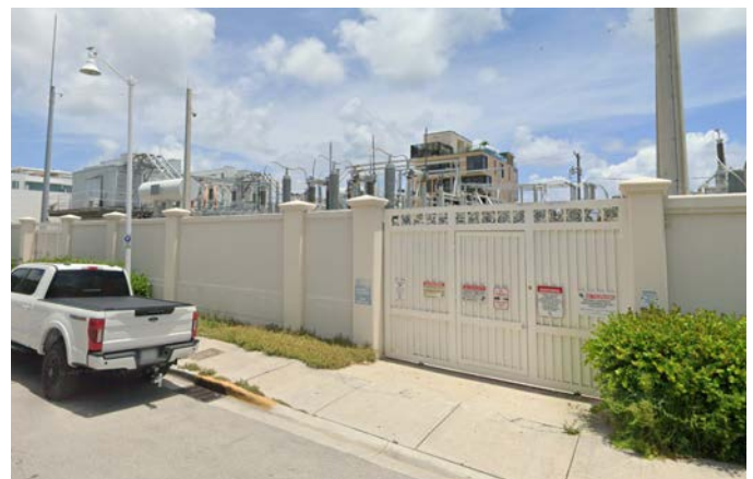
Electrical substation, Source: Google Maps Street View
