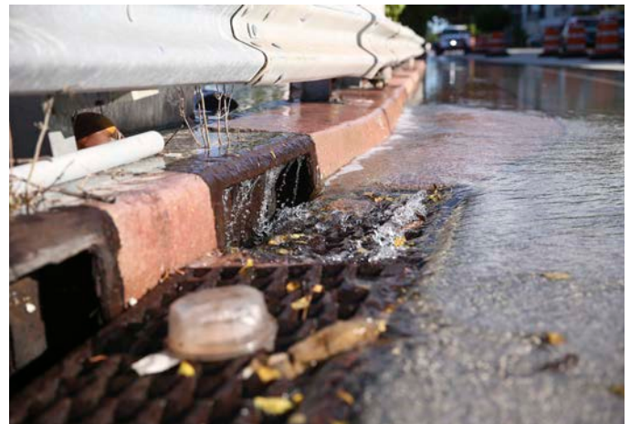
Runoff entering stormwater system in Miami Beach. Source: Miami Beach
