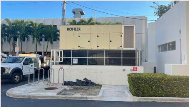
Elevated generator for Facilities building, Miami Beach. Source: Miami Beach
