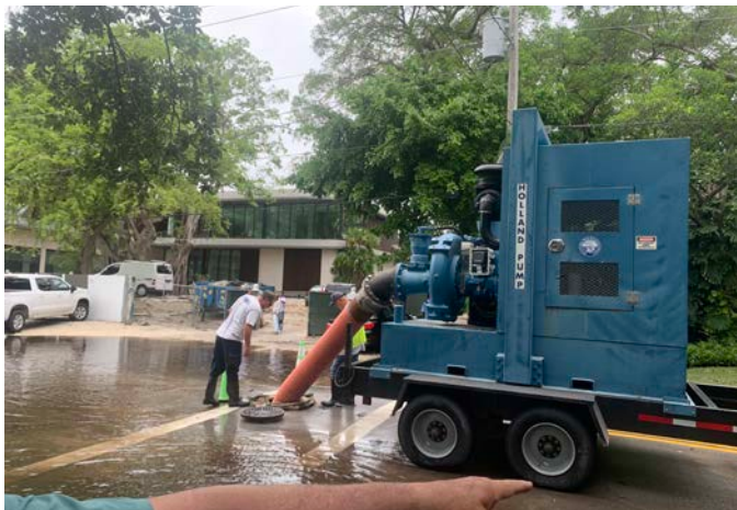
Temporary stormwater pump used to clear floodwaters during June 12, 2024, rain event. Source: Miami Beach
